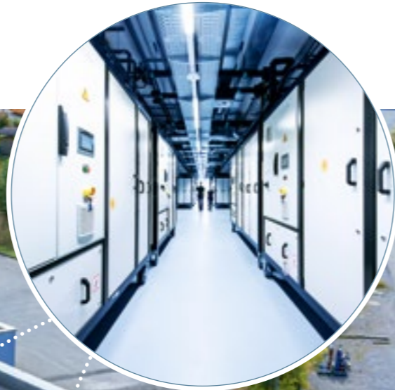
Battery testers and battery heating/cooling systems
